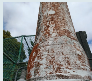
Deteriorated light poles
